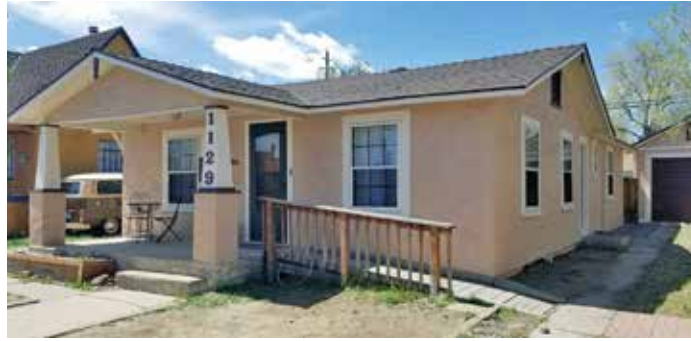
1129 S. Arlington after stucco was patched and repaired and stucco and wood painted.
